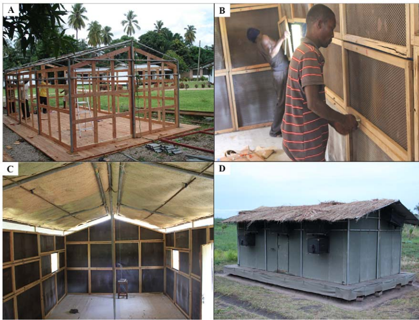
Figure 3. Pictorial representations of selected steps in the construction of the Ifakara experimental huts. Panel A shows the main framework of the Ifakara experimental huts under construction at the workshop. Panel B shows technicians fitting the wall panels, (which are made of chicken wire on wooden frames), onto the inside walls of the Ifakara experimental huts. Panel C shows the inside surfaces of the huts after fitting the chicken wire wall panels and also the palm woven ( mikeka ) ceiling on the underside of the roof, but before the inside walls are covered with mud, and Panel D shows a completed and functional Ifakara experimental hut, fitted with interception traps on windows and eave spaces. It should be noted that the overall shape and dimensions are set to match the typical local houses, shown in Figure 1. The hut is suspended on water-filled metal bowls to prevent predator ants, which would otherwise prey on the trapped mosquitoes. doi:10.1371/journal.pone.0030967.g003
