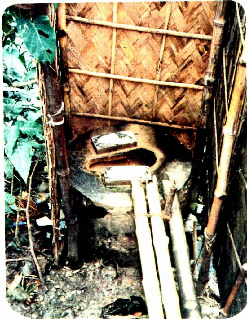
Plate 6. Cemented pan or Pucca latrine (communal)
