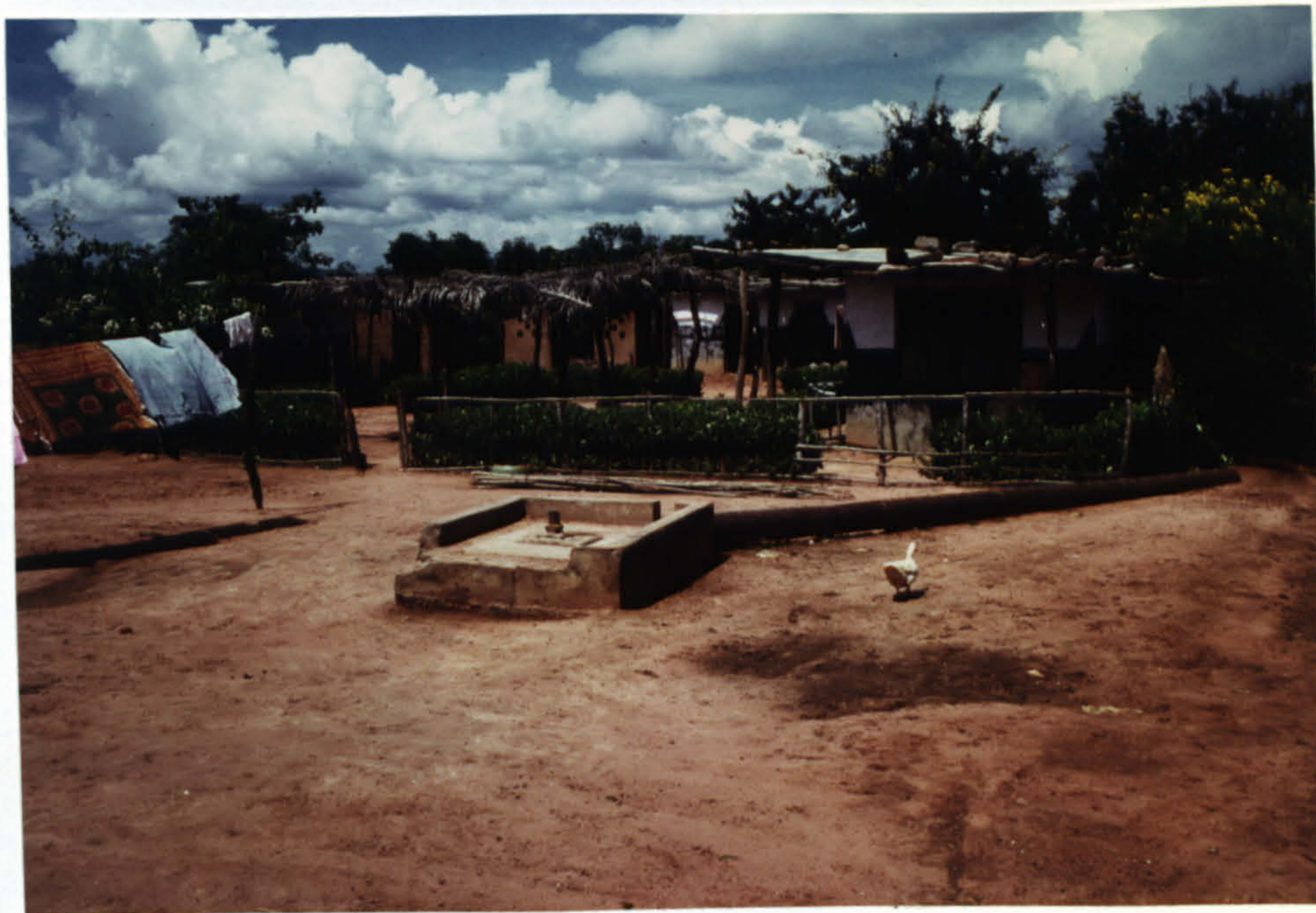
Plate 9. One of three broken WHO project wells at Akokoma, 1980.
