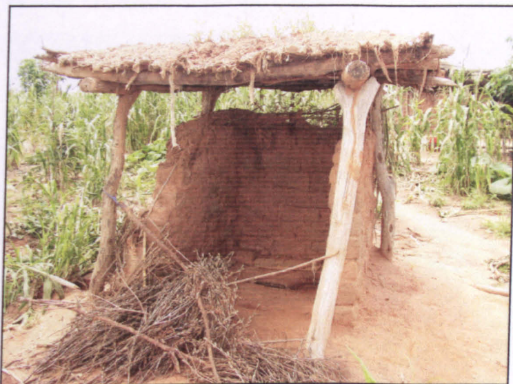
Photo 3.7 Babayu village: roofed latrine with collapsed wall
