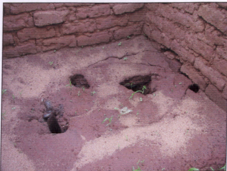
Photo 3.3 Manchali village: latrine showing rain damage to floor
