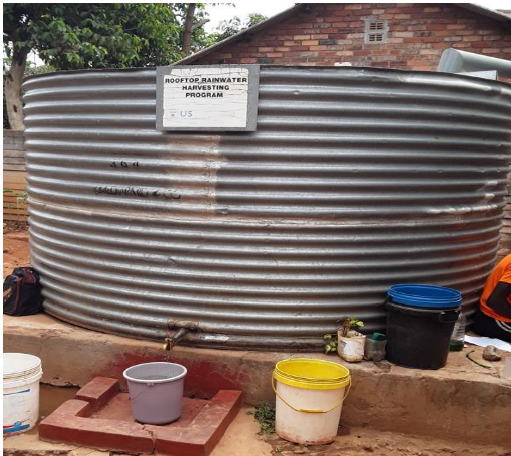
Figure 13: Photo showing Vatete’s rainwater harvesting plant in Mbare
