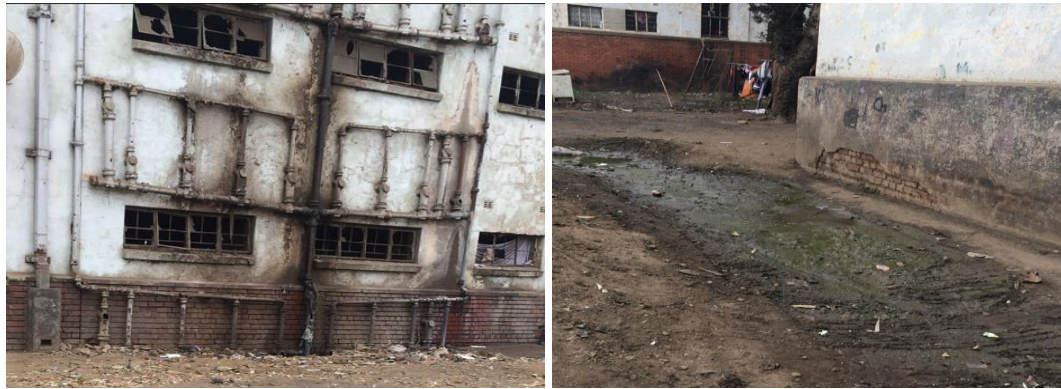
Figure 17: Dilapidated sewers and sewage overflow at the flats in Mbare
