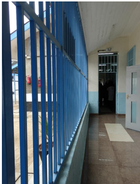
Figure 5.7 Hallway with security bars in the enclosed building of the MAT clinic (EC)
