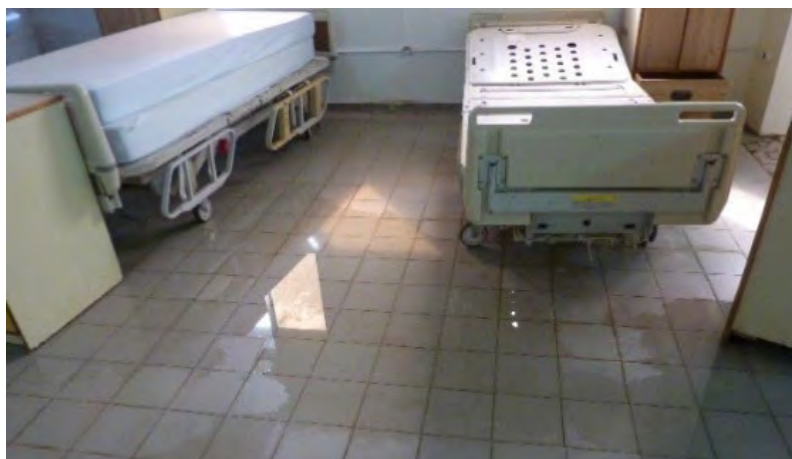
Figure 1-16. Potential KMC unit at EFSTH with flooded floor during rainy season
