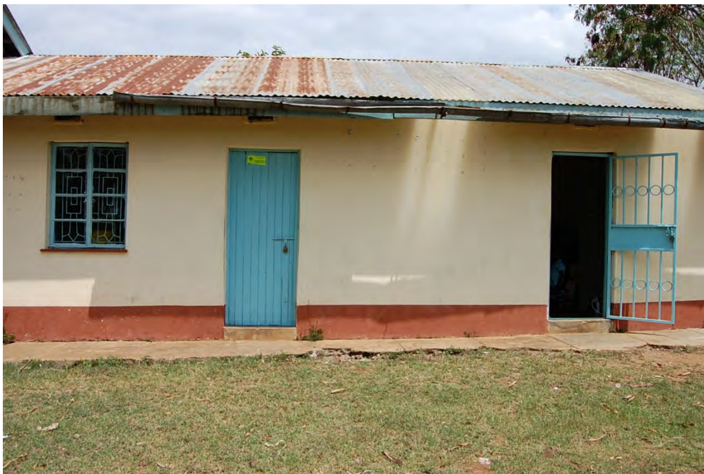
Figure 30: The first building of Nyakogo Dispensary, originally constructed in the mid-1960s. In 2011 this building hosted researchers working with the NCRO/CHA Entomology/Malaria branches. Source: Gemma Aellah
