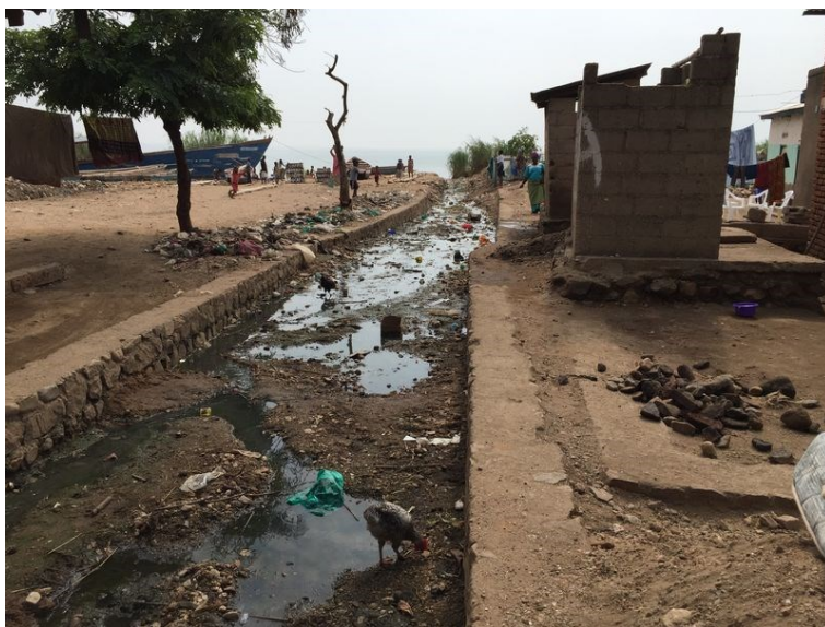
Figure 6-21 An open drainage channel in the Rombe 2 neighbourhood
