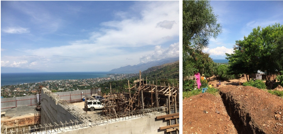
Figure 2-12 Construction of a new reservoir on the hills of Kiyaya overlooking northern Uvira (left); new water pipes being laid in Kasenga neighbourhood (right)
