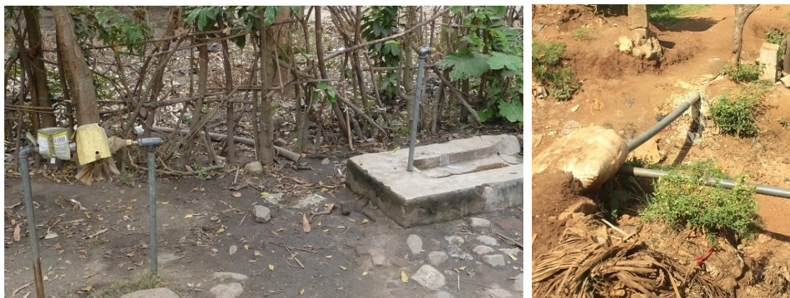
Figure 2-11 Typical tap connection with the tap protected by a lock and meter by a plastic cover (left); exposed water pipe following soil erosion (right)
