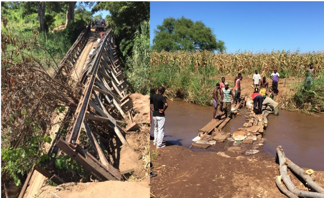
Figure 8: Photos (by the author) showing the broken road bridge on the way to Makanjira from Mangochi (left) and the temporary bridge being constructed by local people a few hundred metres down the river (right).
