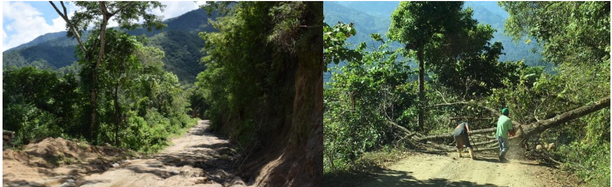
Figure 1-5. A road between two communities damaged as a result of the rainy season (left) and photo of a fallen tree across a road (right) (Photo credit: Georgina Miguel Esponda)
