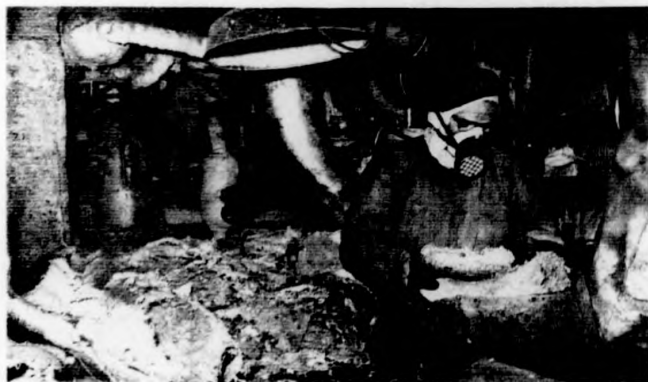
FIGURE 2.8: Asbestos debris in a boiler room.
