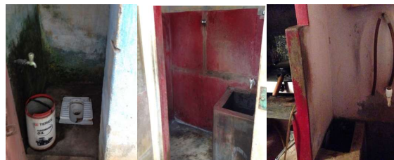
Figure 3.6 Improved water, piped on-premise. The village-level water distribution system pipes water to three taps in each household. MANTRA requires one tap to be placed in the toilet (left), and one in the enclosed bathing room (centre). The household decides where the third tap is placed, but it is typically located in the kitchen (right). Photos: M. Delea
