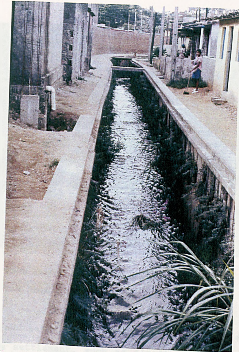
Photo 3. A channel of the stairways drainage system in the Bom Juá neighbourhood
