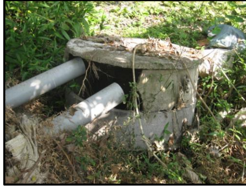
Figure 8. Broken latrine pit in Kajisahi village
