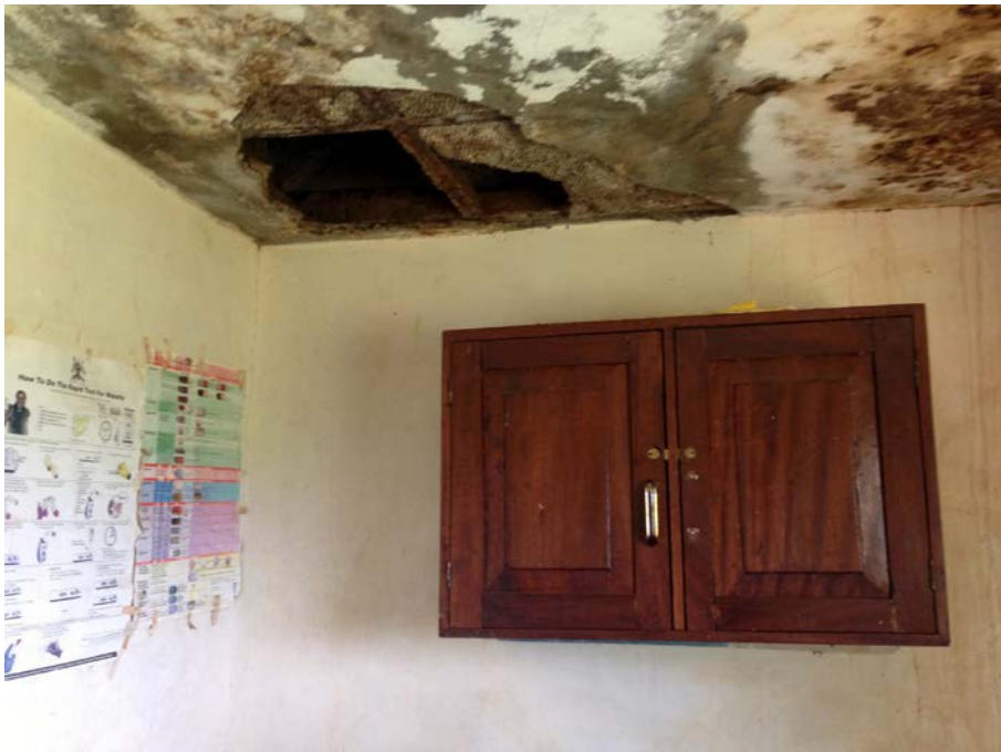
Photo 7.3: Health centre 10 – Damaged ceiling
