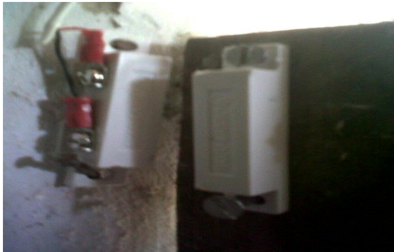
Figure 5-15: The door switch installed in latrines during the Phase 2 pilot testing in Bhoigun, rural Odisha, in June 2012.
