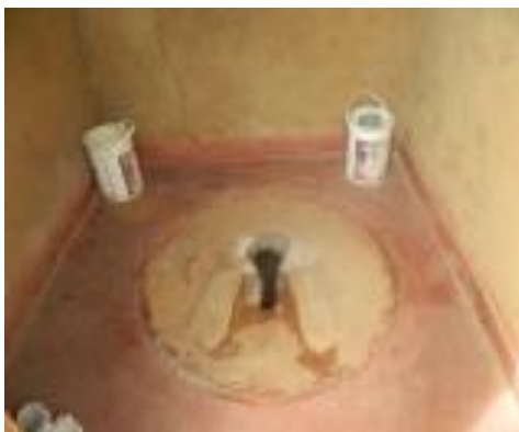
Figure 5.3: Pit latrine with a slab/cement floor
