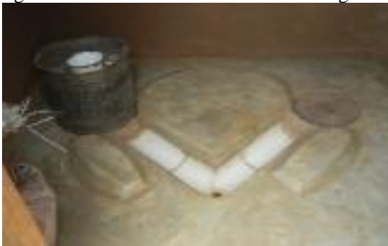
Figure 3. 1: Interior view of urine diverting toilet
