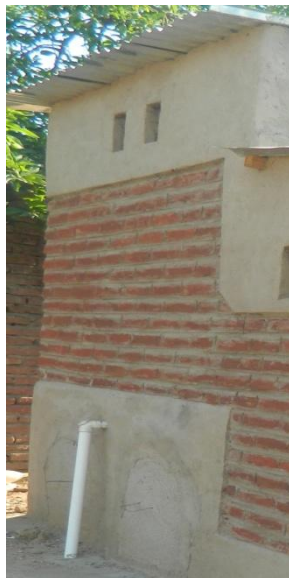
Figure 7. 2: UDT pipe for diverting urine into soak pit
